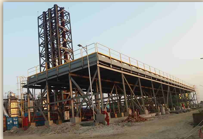
Radiator & Stack Tower
