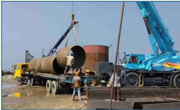
Exhaust duct transportation
