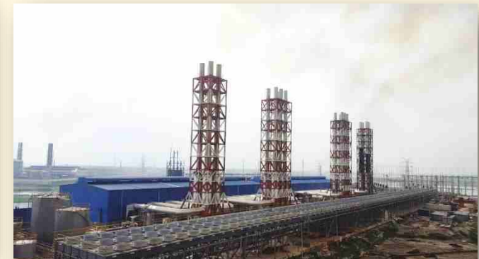
Radiator & Stack Tower
