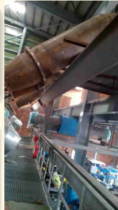
Charge air duct
