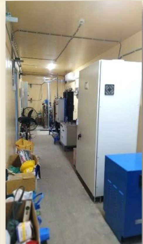
H2 plant Inside equipment
