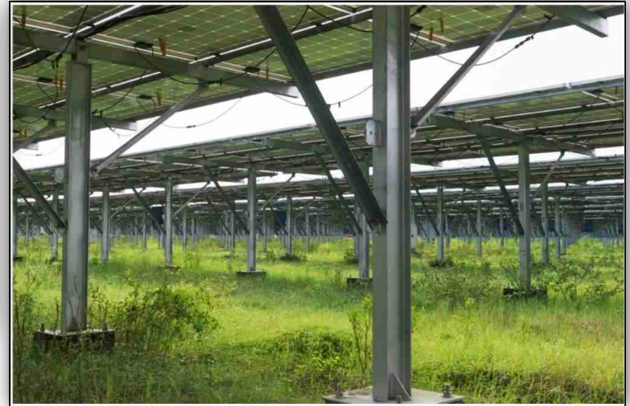
Solar Panel Structure
