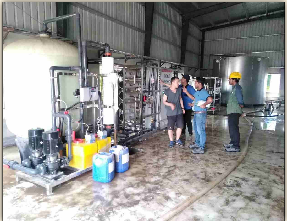
WTP - 24M 3 /Hr Capacity (Summit Group, Gazipur)
