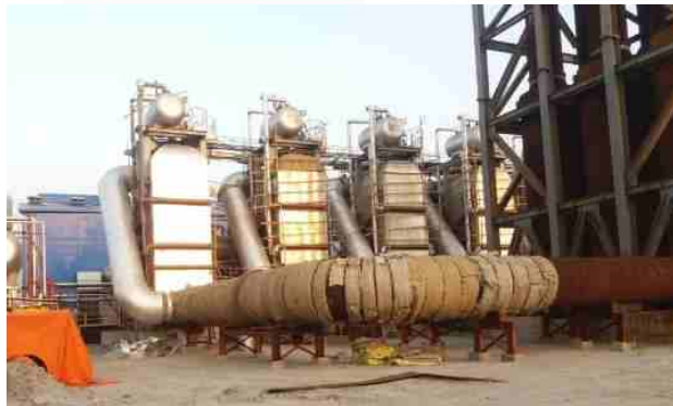
Exhaust duct Insulation
