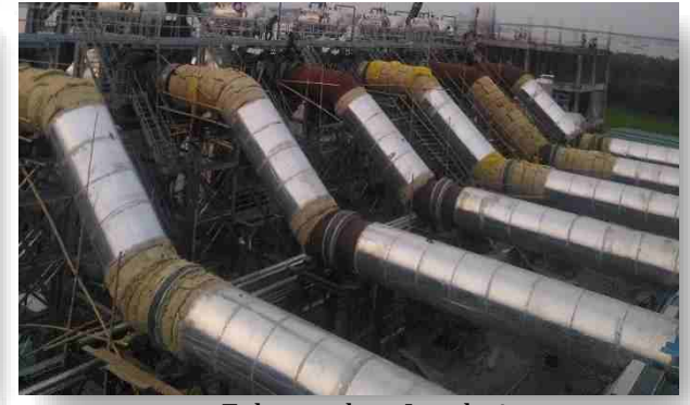
Exhaust duct Insulation
