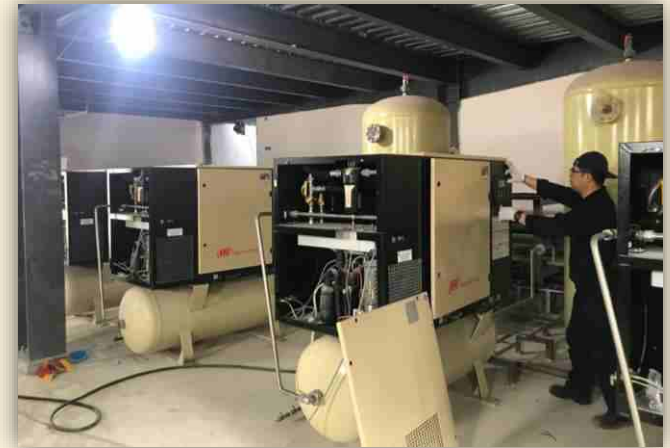
Instrument Air Compressor (IR)
