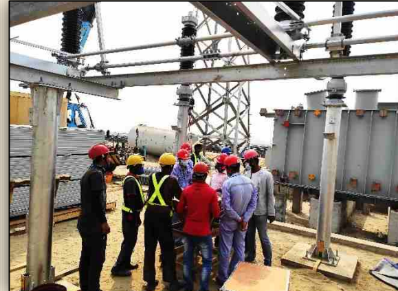
Substation Testing and Commissioning
