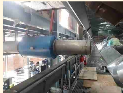
CA Silencer Install
