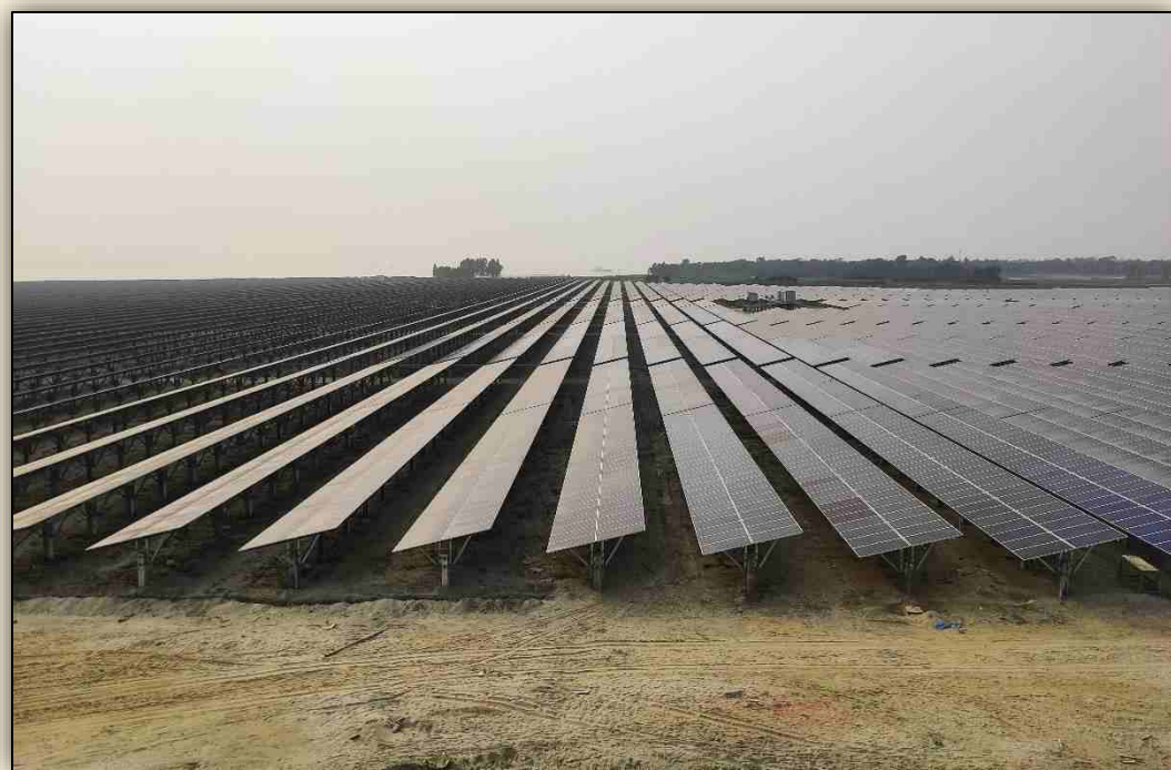
MMS and PV panel
