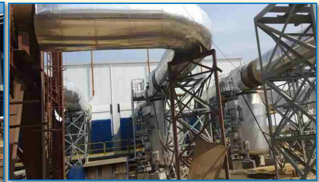
Exhaust duct support
