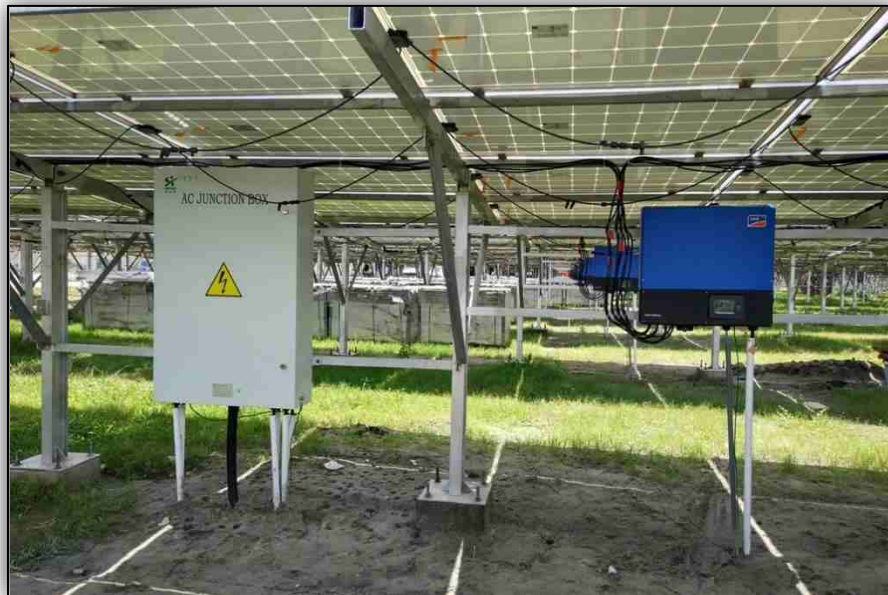
Solar Panel Board
