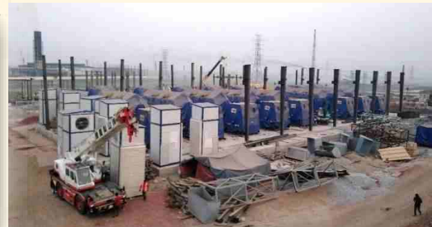
Alternator Hot air Duct
