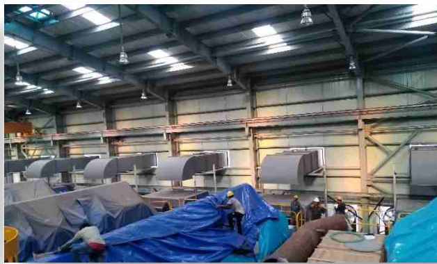
Alternator Hot Air Duct
