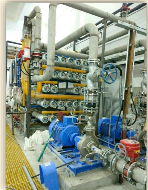
Water Treatment system
