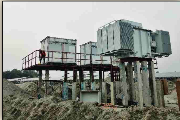
Inverter and Transformer
