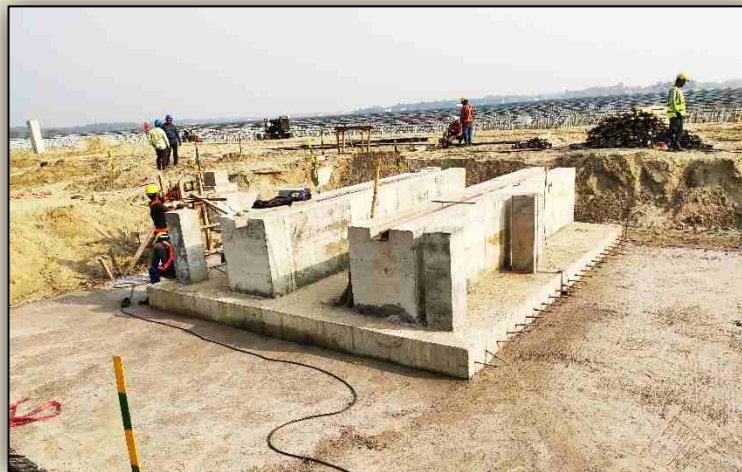
Main Transformer Foundation
