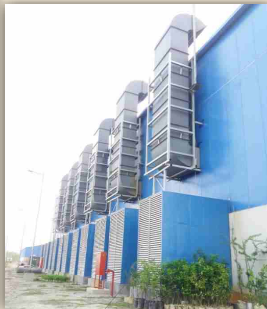
Alternator Hot air Duct
