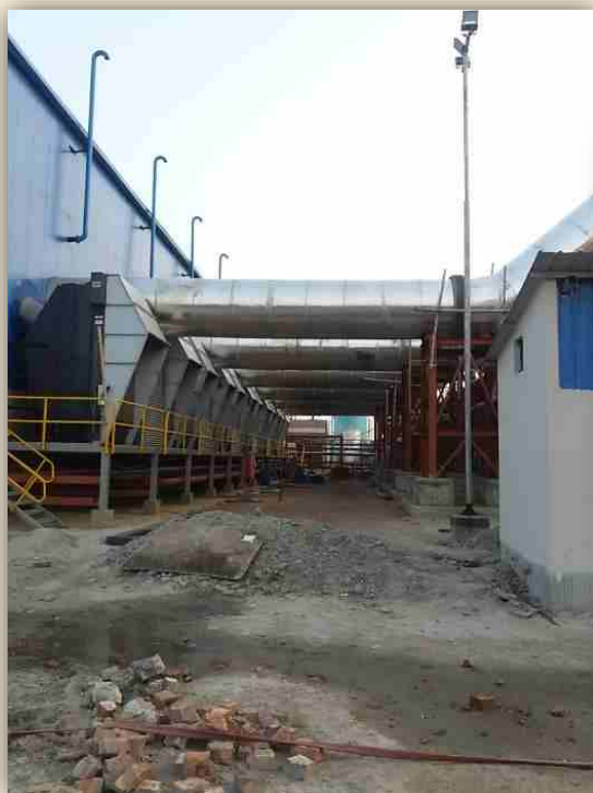
Radiator & Stack Tower
